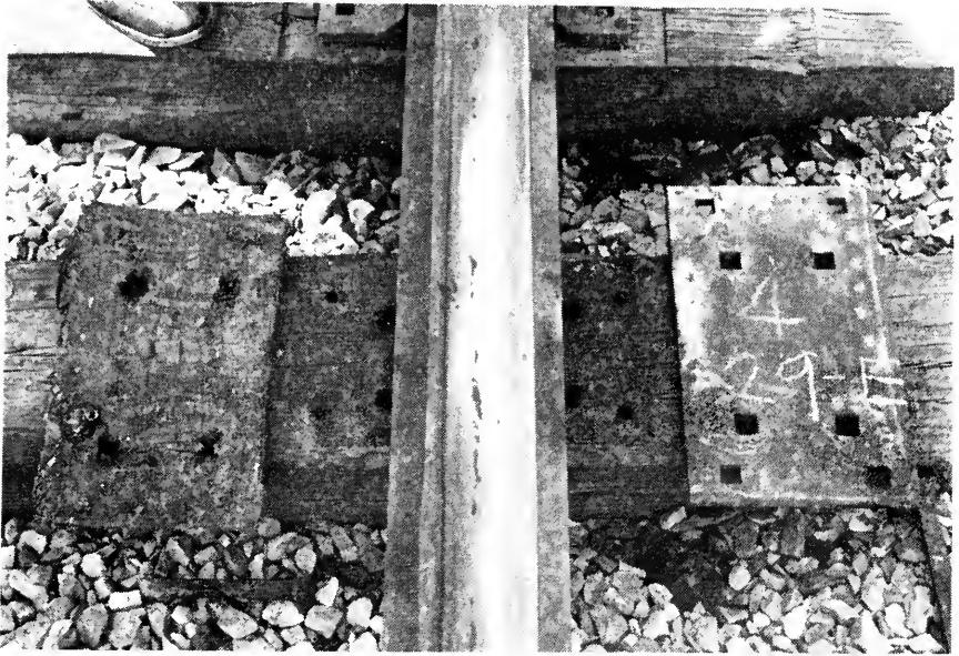
Fig. 18. South Portion Section 1, 1-in Bird 7-ply Duck-Barlap Tie Pad. Coated. After 71 months' Service to the Inner Rail of the Long 4-1/2° Curve.
